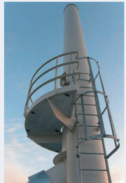
Flue gas stack with emission control device
